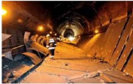
(Photo of ceiling collapse accident in Sasago Tunnel on the central expressway)
